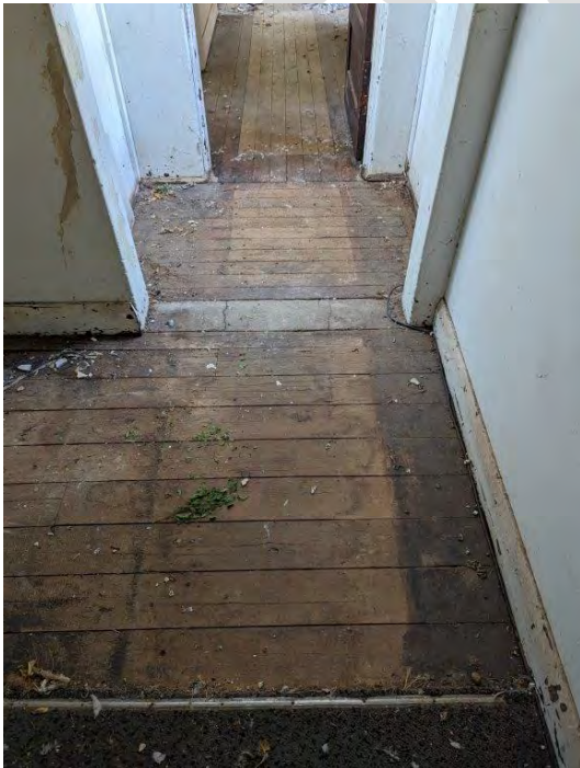
Photograph 141 The junction between the main wing and the link over into the extension wing. A separate stair leads off to the left to serve as the separate escape from the main Castlereagh wing.
