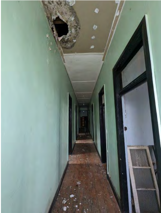
Photograph 136 View looking back north along the hall, noting the ceiling damage (also shown in photograph 128).
