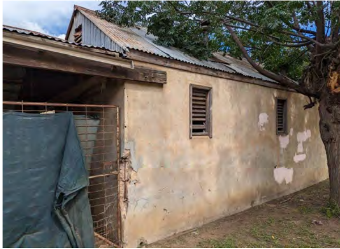
Photograph 23 The West elevation facing into Skillman’s Lane noting overgrown tree, damaged roof, missing gutter and damaged corner of wall. These elements appear capable of restoration while the attached roof to the left is an extension and has minimal significance.
