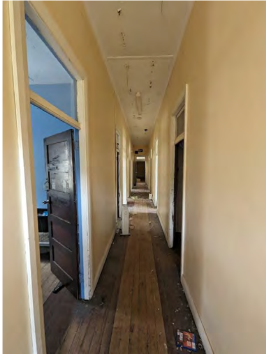
Photograph 146 A general view looking east, noting the pigeon damage due to a major infestation through open windows on the southern side of the wing.
