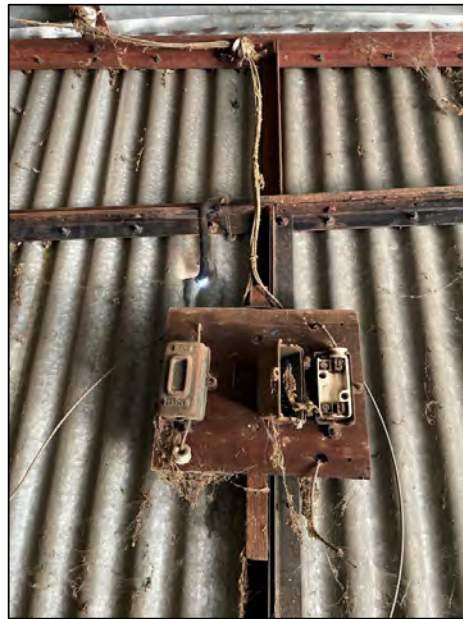
(2) Carport, internal, original wiring presumed positive. Further investigation is required
