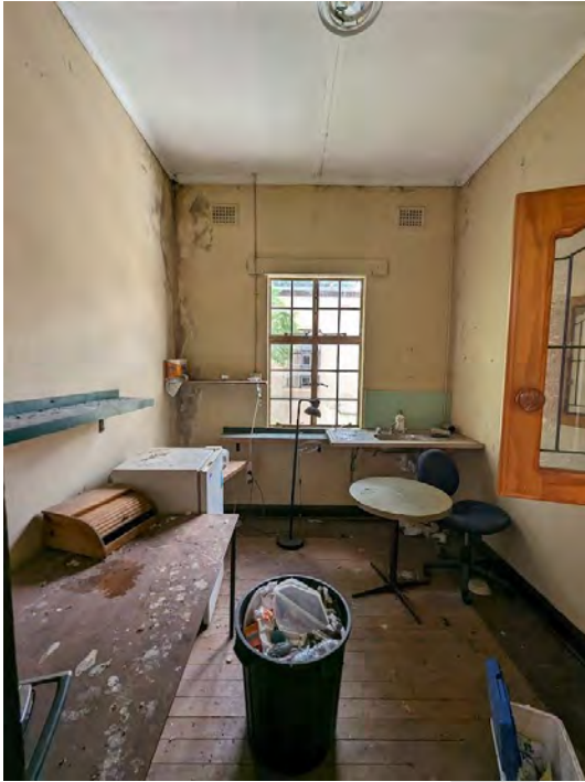
Photograph 148 The end room on the north side, noting the poor condition.
