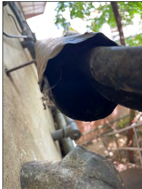
(12) External, sheathed pipework
