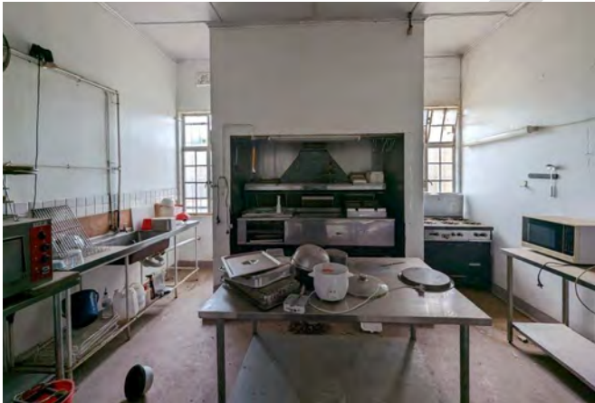
Photograph 72 View of the general layout indicating that the equipment is generally sound and could be serviceable.
