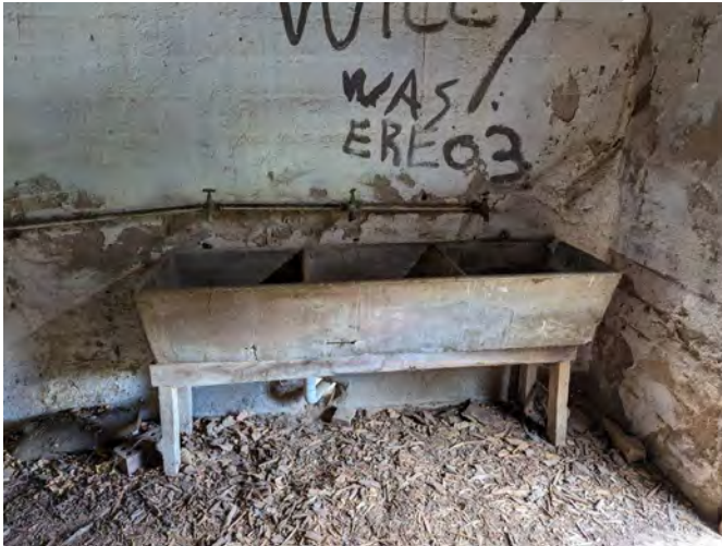
Photograph 29 Alteration for laundry trough installation
