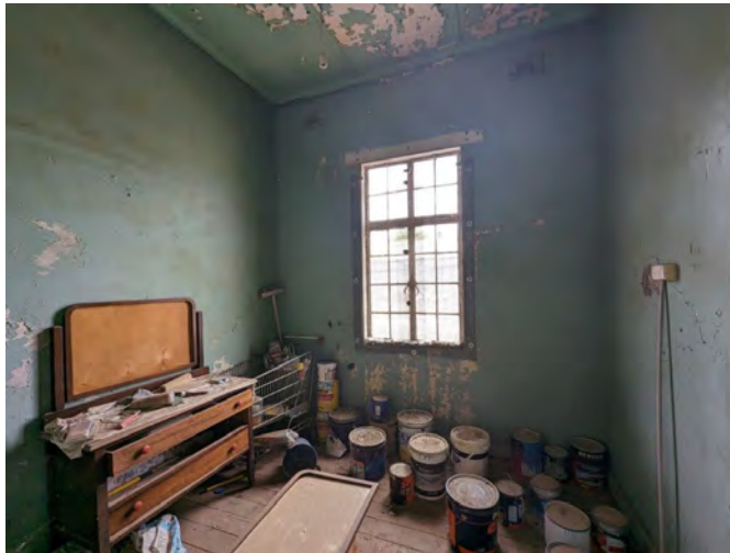
Photograph 80 Typical room on the northern side of the north service wing with window to Skillman's Lane.
