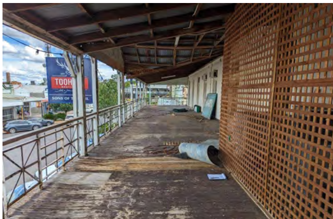
Photograph 59 A general view noting lattice screening for the air-conditioning systems installed on the verandah. It is likely that condensate has damaged the flooring.
