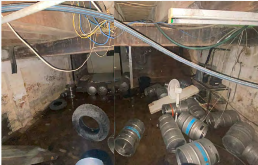
Figure 26: Water ingress into cellar. This will deteriorate timber members and corrode steel members. In addition, this will damage masonry structures.
