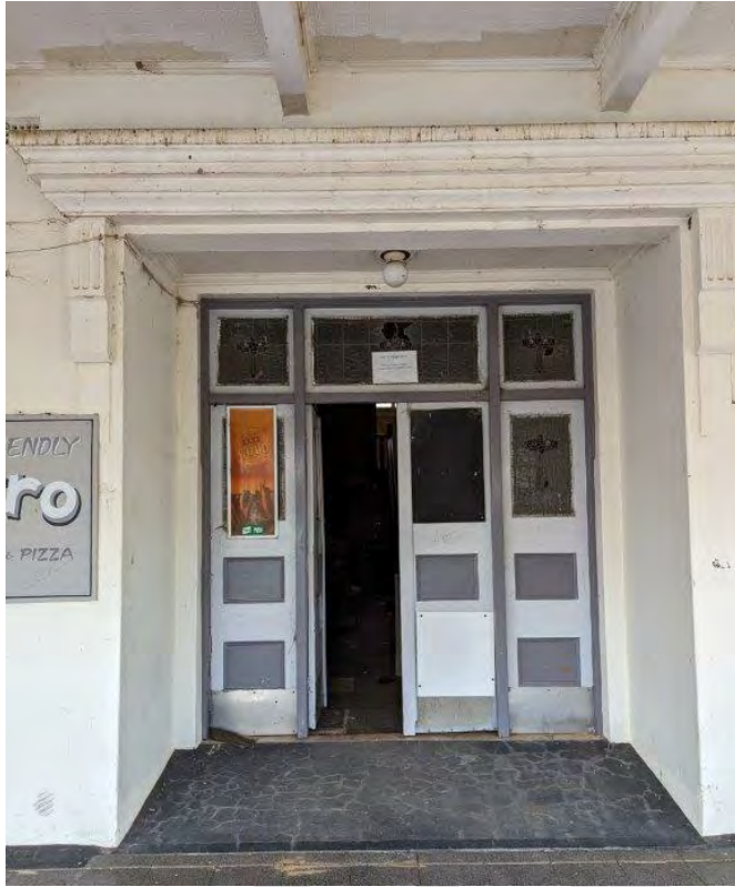
Photograph 19 The Guest entry to the lobby retains the original features with only minor reinstatement & restoration required. The entry is accessible.
