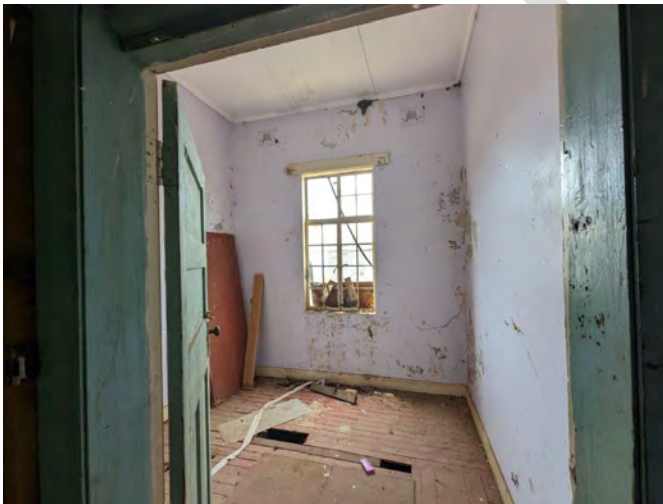
Photograph 77 A room in poor condition on the northern side of the North wing.
