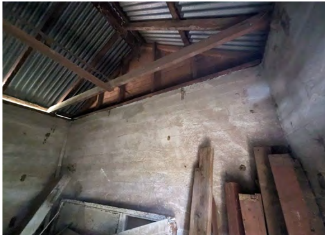
Photograph 25 An internal view of the walls and roof structure, noting the generally sound condition.
