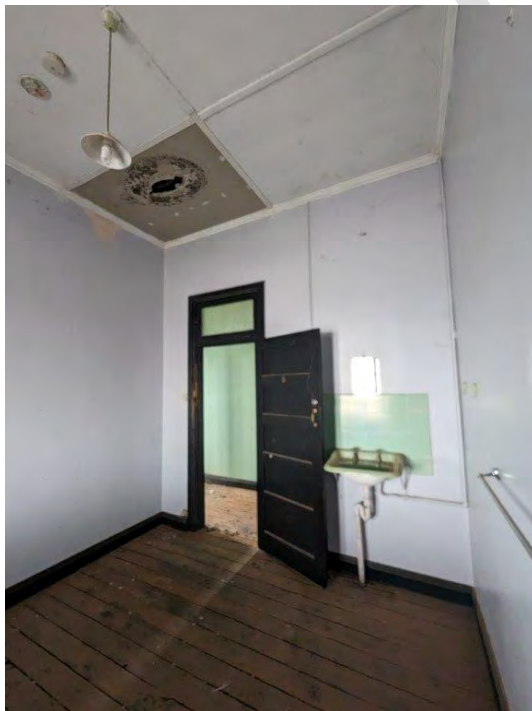
Photograph 131 Internal view of Room No.9 noting ceiling damage.
