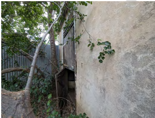
Photograph 24 View within the overgrown area of the south western corner of the stable and southern boundary steel fence.
