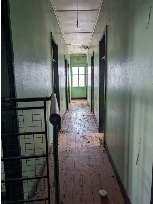
Photograph 128 General view looking south to the end of the wing, noting the ceiling damage and pigeon infestation.
