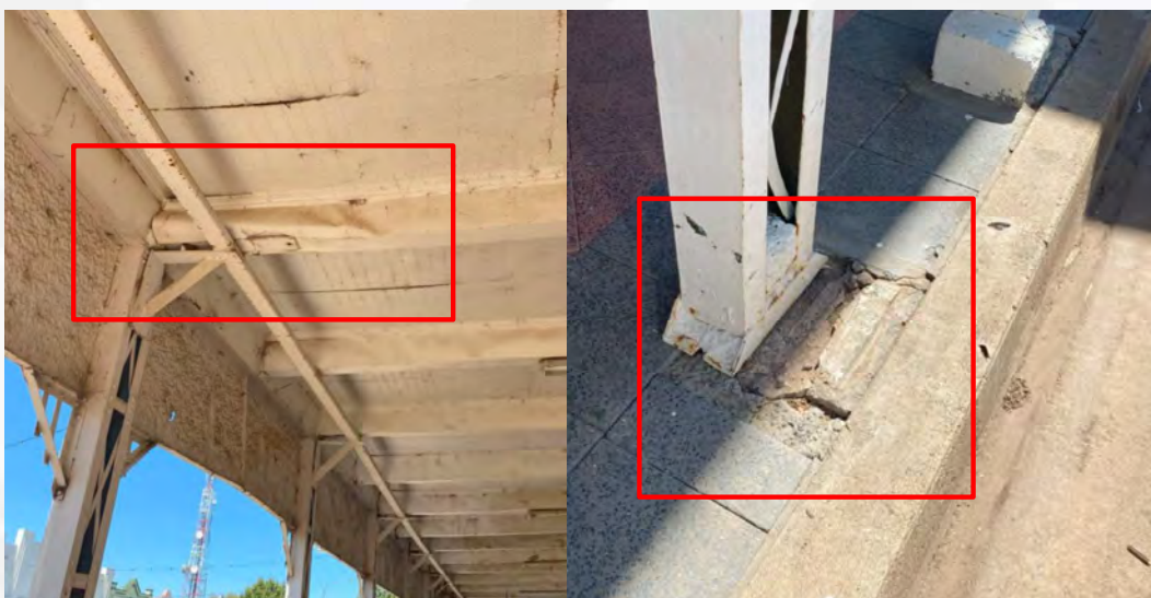
Figure 22: A number of floor beams were observed to be broken. Column displaced from footing. Structure may be unstable.
