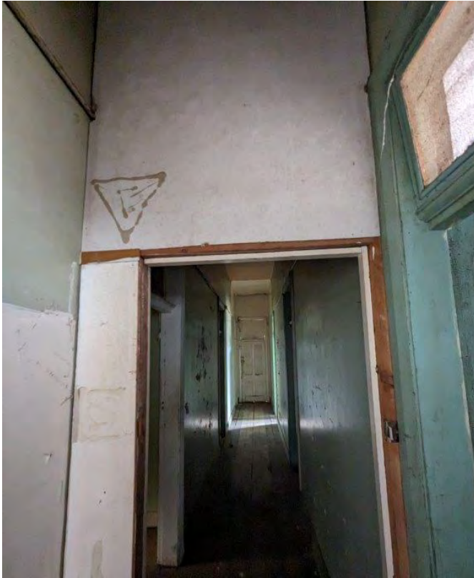
Photograph 78 View from the kitchen end towards the staff rooms and the separating partition.
