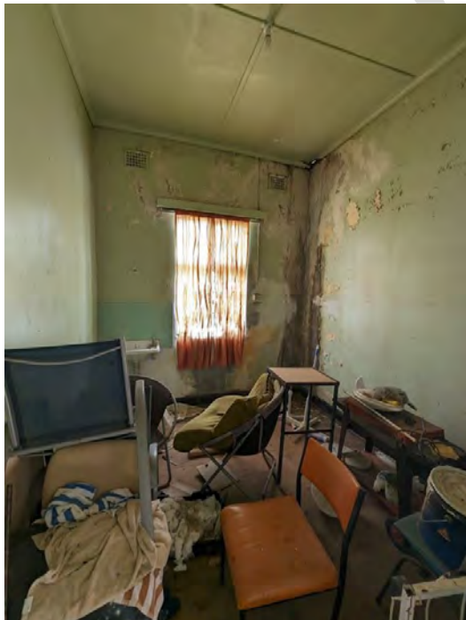
Photograph 147 View of the room interior, noting the condition. The room size is smaller than the original rooms. The condition is poor with damage due to roof leaks. It appears that this wing has not been utilised for some years for guest accommodation.
