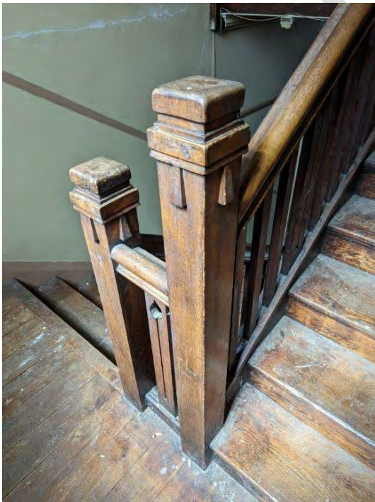
Photograph 99 A detail view of the central newel post at the middle or half landing.
