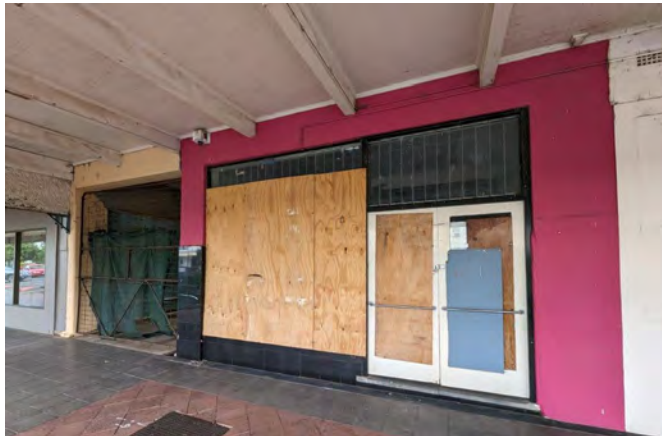
Photograph 13 The drive through bay and then the former separate retail shop unit. The tiled area and glazing are contemporary and not sympathetic with the original. Suitable tiling and shopfront may be reinstated within the opening.
