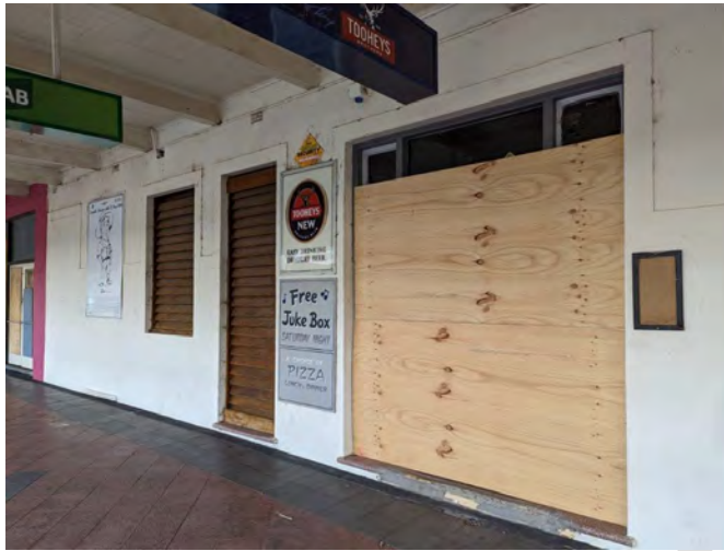
Photograph 16 View of the main entrance to the bar. The details of the doors and sidelight panels are generally intact with minor conservation works to the glazing.
