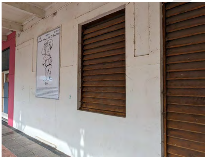
Photograph 14 The window and door openings have been modified as part of meeting the smoking requirements. Suitable replacement doors and windows could be reinstated.
