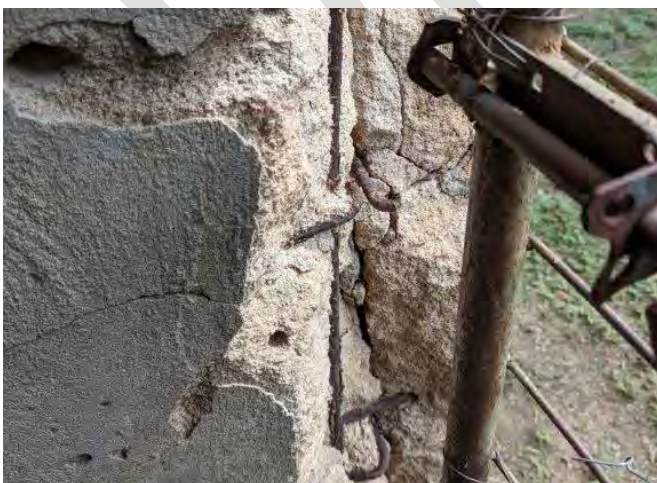
Photograph 32 The damaged North west corner, noting the reinforcing forming part of the concrete wall construction.
