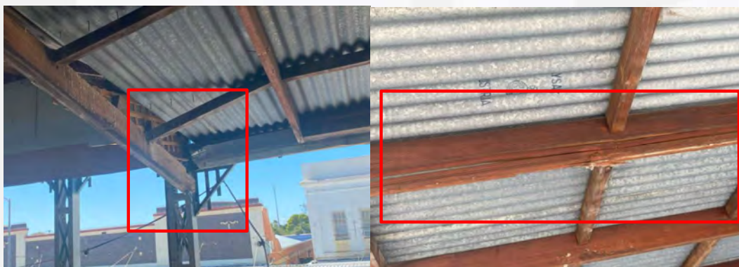
Figure 21: Broken roof members on balcony. Structure may be unstable.
