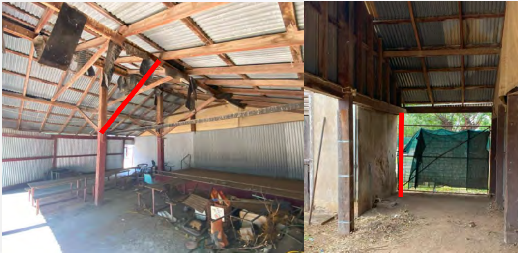
Figure 24: Missing members from outdoor timber structure. Structure may be unstable.
