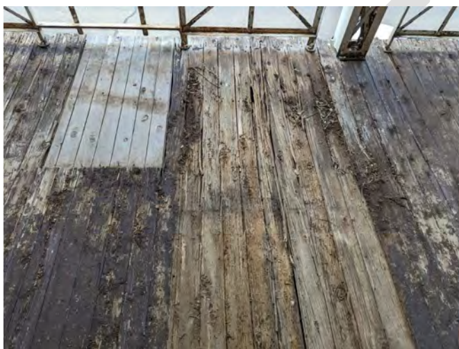
Photograph 60 A close view of damaged flooring & part replacement floorboards near the AC installation.
