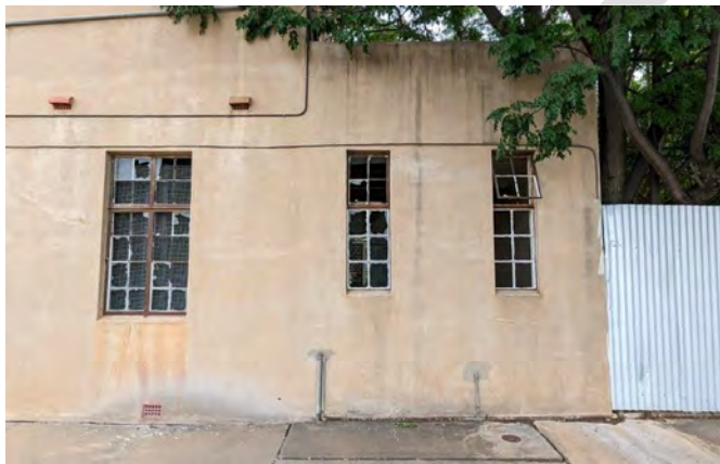
Photograph 52 The small single storey room at the north western corner is the laundry. The overgrown tree requires removal to reduce the impact of the roots on the building.
