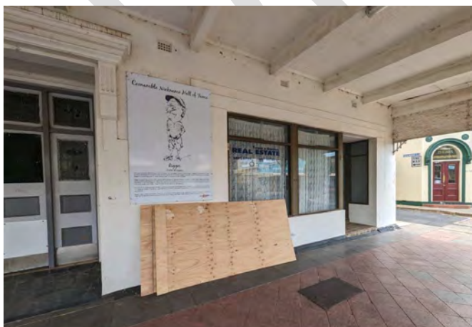
Photograph 20 The end of the elevation indicates the second retail shopfront which is a replacement for the original door and two windows. A suitable replacement could be provided for the uncharacteristic aluminium units.
