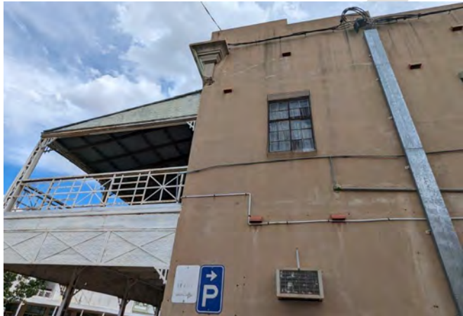
Photograph 49 The North elevation of the eastern end of the north wing, noting the returning faced detail, the attached verandah and services applied to the wall.
