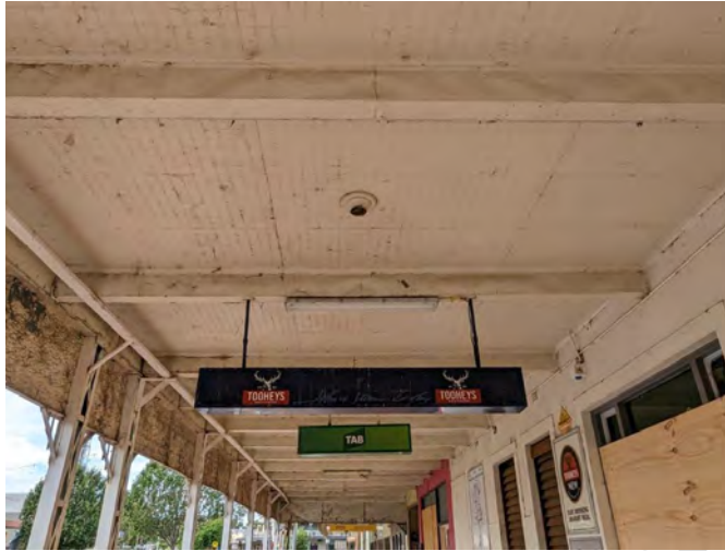
Photograph 11 A view of the pressed metal verandah soffit, looking south, noting earlier light fittings and the later steel brackets & batten on the posts
