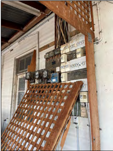
(33) 1 st floor external deck switchboards
