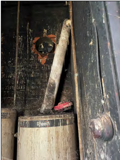
(15) Internal, boiler room pipework
