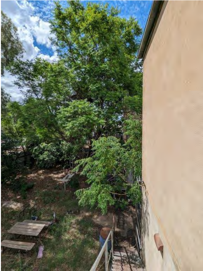
Photograph 37 View from the fire stair on the central wing looking north west down to the rear yard. The overgrown tree next to the wall requires removal to reduce the impact of the roots on the building.
