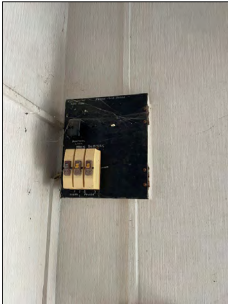
(35) Former travel agent, internal, switchboard
