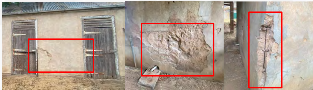
Figure 25: Reinforcing steel has corroded and is breaking concrete away as it expands. Structure may be unstable.
