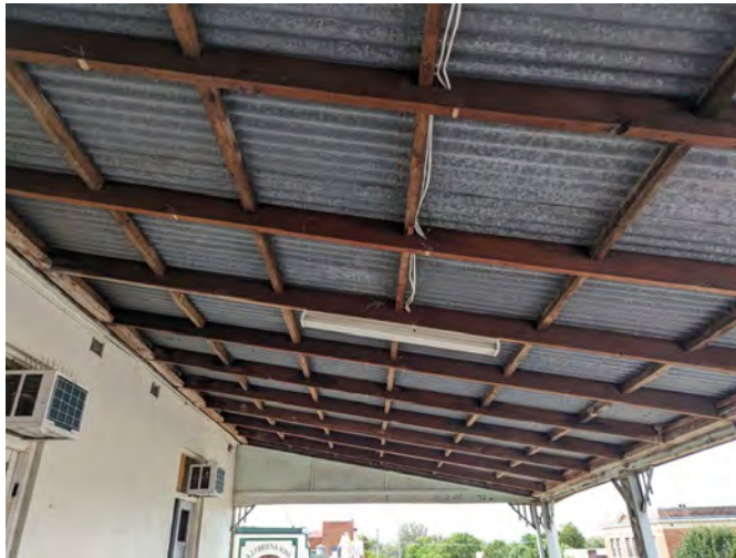
Photograph 57 The roof structure towards the northern end of the verandah. Traditional lighting can be installed.
