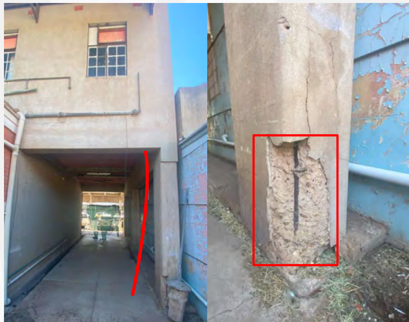
Figure 20: Columns at the southern end of the building are beginning to buckle with concrete breaking away from reinforcement. Structure may become unstable with more soil and building movement.
