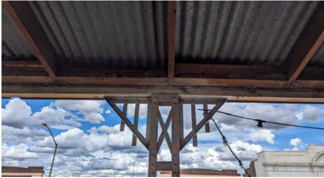
Photograph 62 An example of a typical fabricated steel bracket to the verandah structure. The steel is worthy of a structural review but appears sound and can be restored with a clean and paint.
