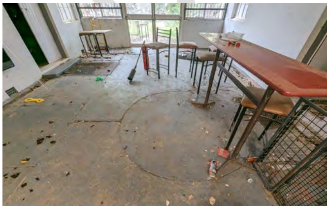
Photograph 94 The circular concrete lid is suspected of being the cistern where the stormwater was stored.
