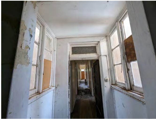
Photograph 142 View looking west to illustrate the bridge link between the Castlereagh wing and the extension wing.
