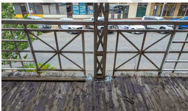
Photograph 61 A general view of the flooring and balustrade. As the gaps within the balustrade do not comply with the BCA, an additional mesh screen or similar plus top rail will need installation for compliance.
