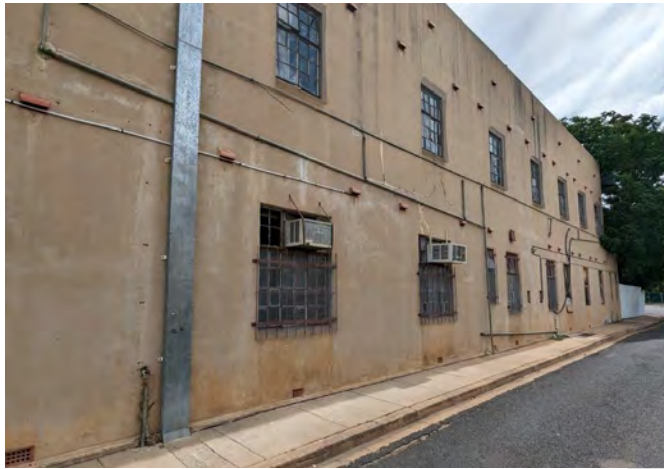
Photograph 51 View of the North elevation, looking west, noting the extent of glass repair required to the windows
