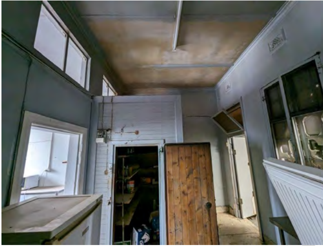
Photograph 74 View of the cool room which was installed within the original room layout. The kitchen is to the left and courtyard to the right.
