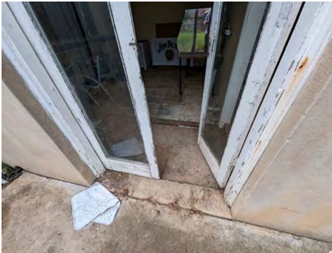
Photograph 33 The door set in the ground floor at the west end of the wing, noting the water damage and lower floor level
