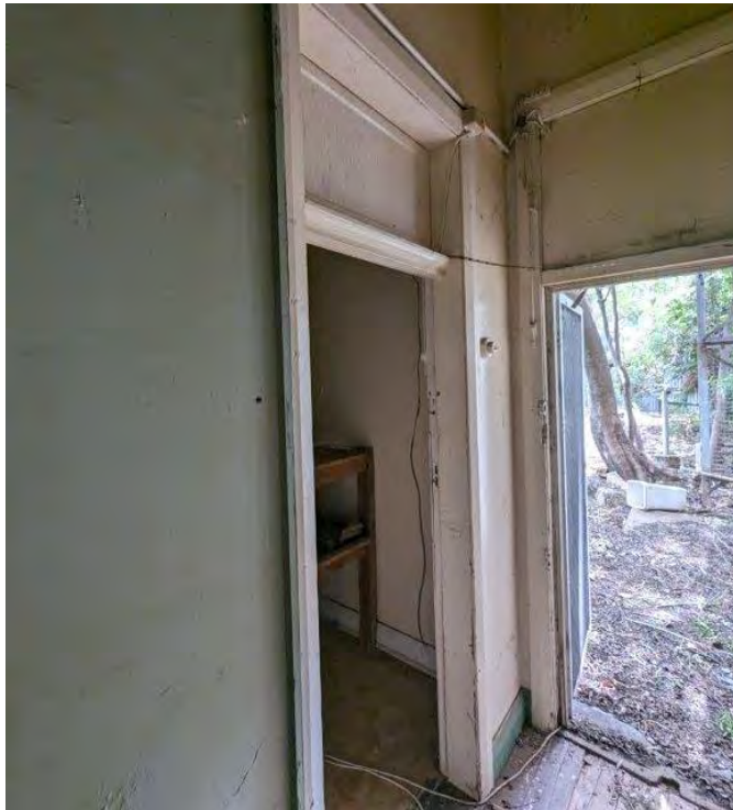
Photograph 82 View of the rear exit door and door to the courtyard side rooms. Note the levels which allow water to enter the building. This can be addressed by reducing the external level and introducing a step for Code compliance (weatherproofing).
