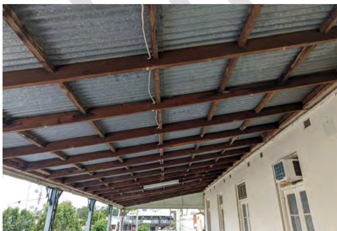
Photograph 56 General view of the verandah roof structure towards the southern end of the structure. The structural capacity is to be reviewed.
