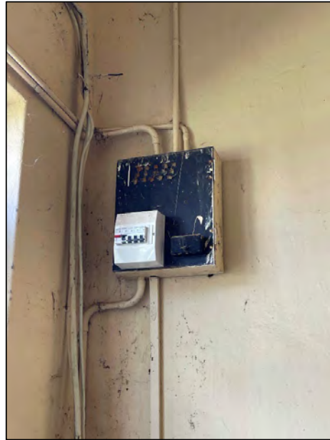
(14) Internal, outside bar switchboard
