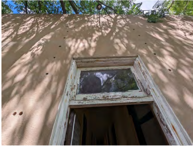
Photograph 41 A view of the wall construction from the fire stair noting the rod holes left from the reinforced wall construction.
