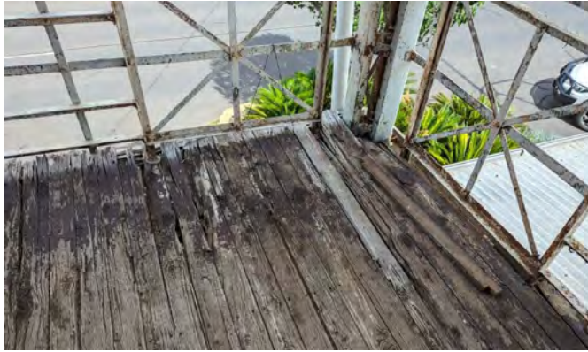
Photograph 54 View of the poor condition of the cypress tongue and grooved timber flooring on the verandah at the south eastern corner. The greater level of exposure has caused the greatest deterioration.
