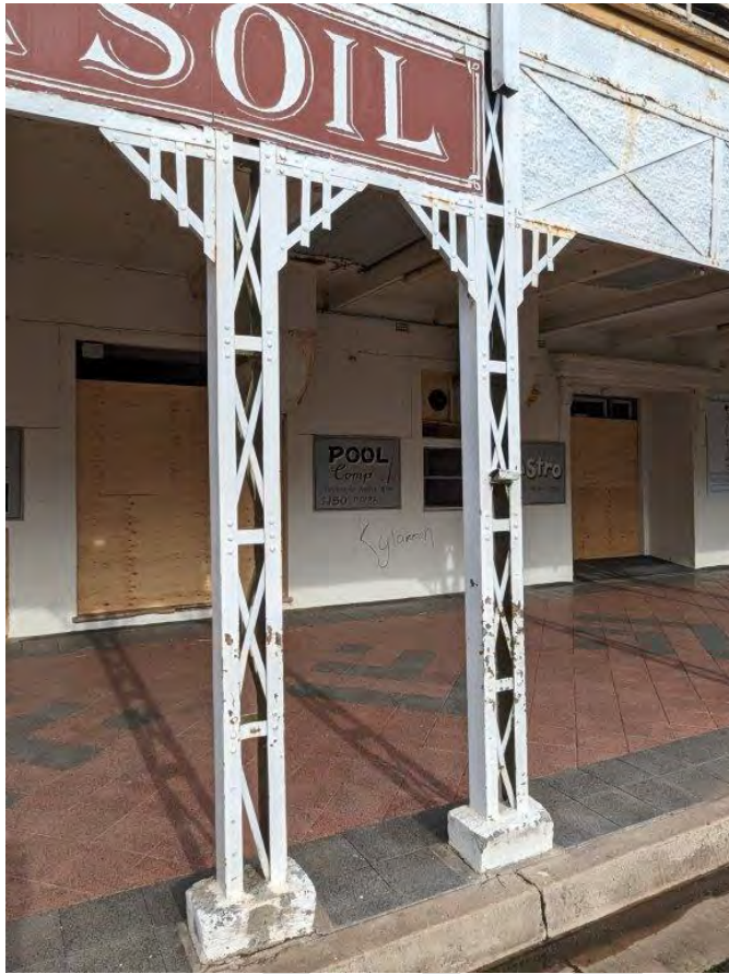
Photograph 10 A close detail of the verandah post steel structures, bases, decorative brackets and roughcast finished infill sheets with diagonal braces. The downpipes are missing.
