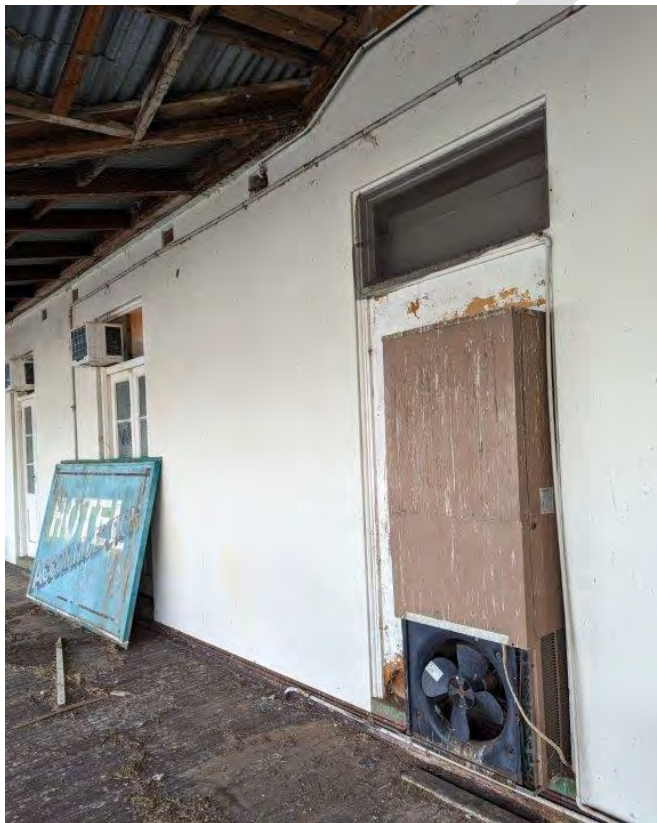
Photograph 58 Air conditioning systems for the bar in this central area have damaged the front elevation which can be restored.
