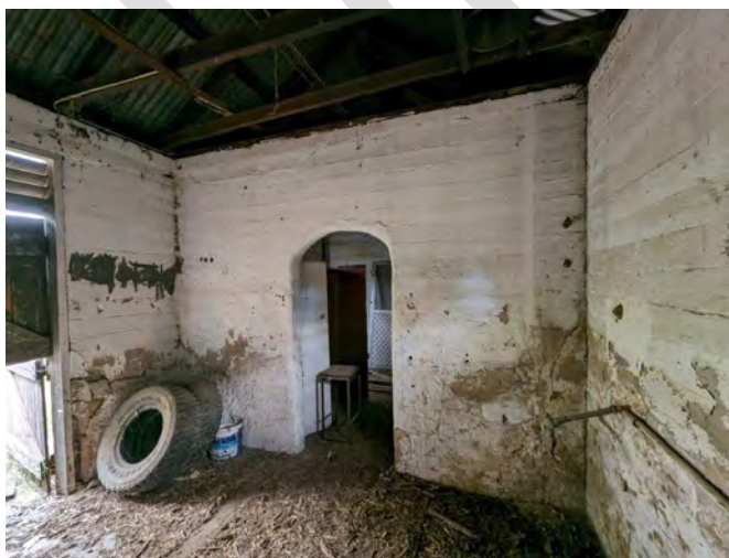
Photograph 27 View of the eastern end noting the arched construction and damaged wall.
