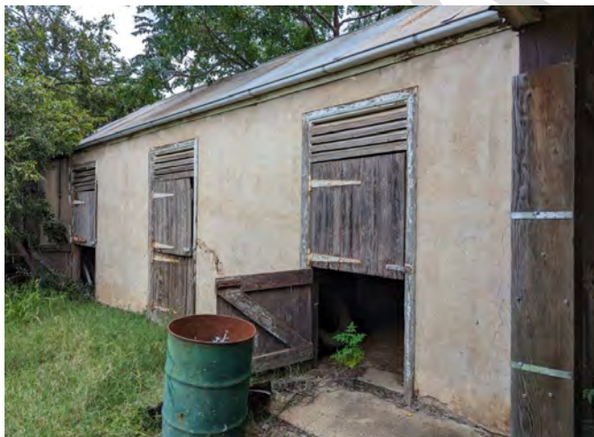
Photograph 22 The East elevation of the stable building which faces into the yard, noting the intact joinery, walls and roof.
