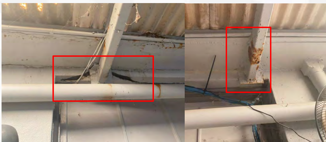
Figure 23: Outdoor roof structure, between the two western wings of the building has detached beams or heavily corroded members. Structure may be unstable.
