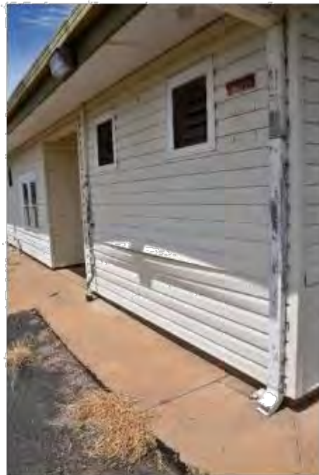
Fix Cladding Repaint exterior and fix downpipes
