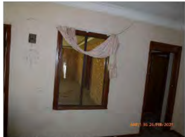
Major Cracking near entrance
