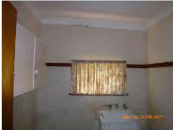
Cracking in Laundry
