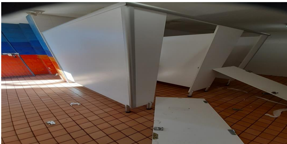
Damaged Male Toilets at Smith Park, Coonamble
