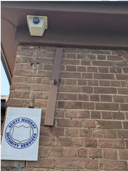
Photo 2 Engineer to advise on long term for tie rods after remedial work complete
