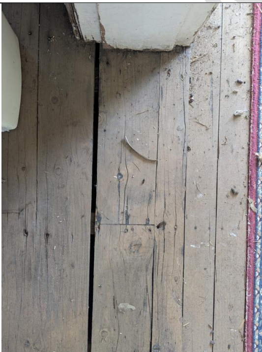
Photo 18 Timber filler strip required following remediation
