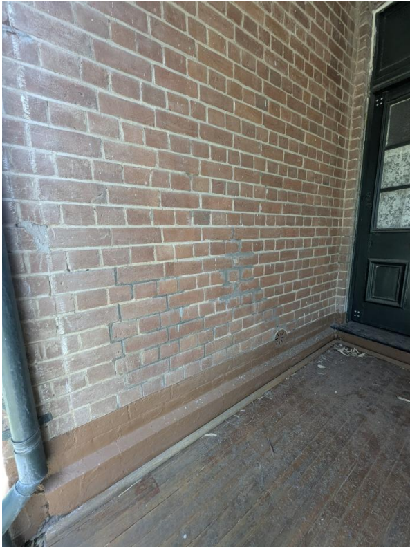
Photo 15 Previous cement repairs to be replaced
