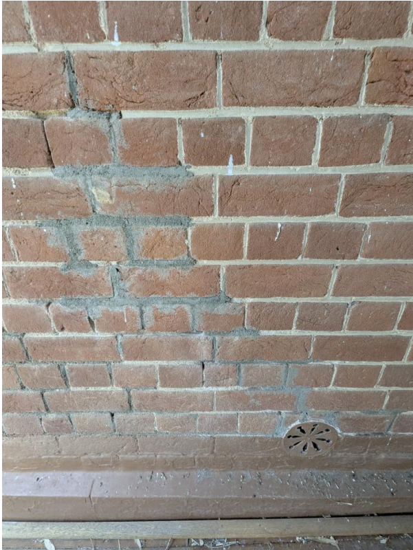
Photo 14 Previous cement repair to be replaced with lime mortar. Sub-floor vents noted
