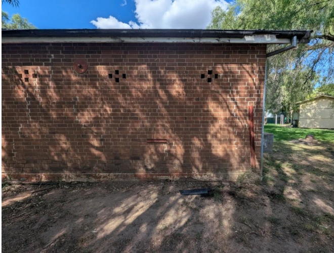
Photo 27 The corner of the significant building which is close to the Stauion, noting the failed guttering.
