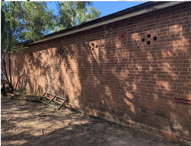
Photo 28 Note the wall cracking evident in the following interiors. Note the wall plates from the cross bracing rods.
