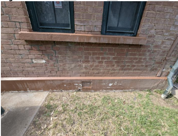
Photo 10 Note general replacement of irrigated lawn within 1200mm of building
