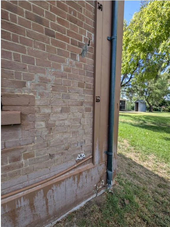
Photo 7 Engineer to advise on bracing system following remedial works
