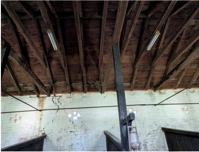
Photo 31 Wall movement cracking. Following ground engineering and the apron extension and stabilisation, the movement cracks can be Helifix brick stitched. The engineer to comment on whether the rod and brace system is to be released to reduce further damage
