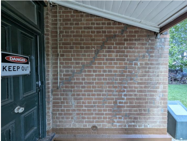
Photo 11 Previous pointing in cement to be replaced with lime-based mortar
