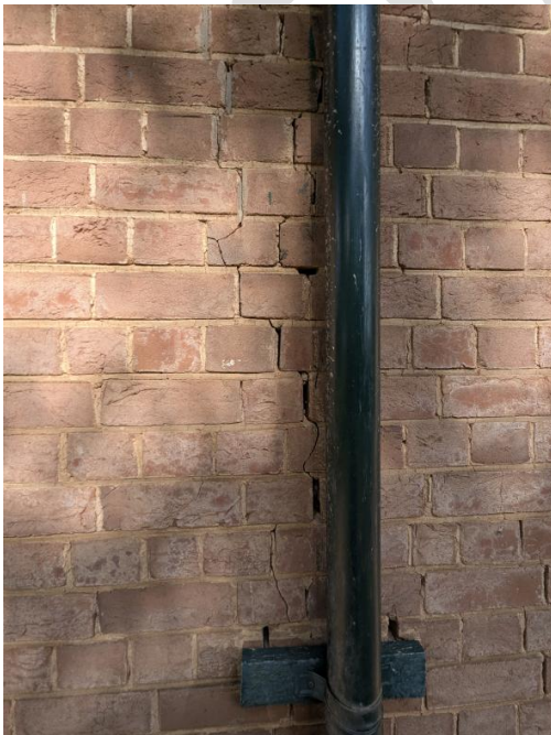
Photo 16 Movement cracking affecting bricks and not using joints
