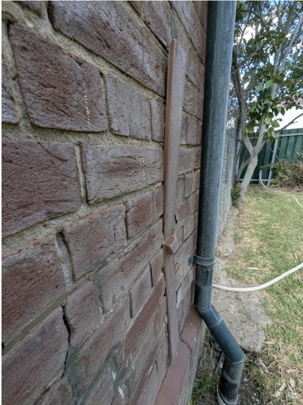
Photo 9 Note that rods in tension appear to have damaged walls after movement: Engineer to advise on remediation – rod retention or removal following remedial work
