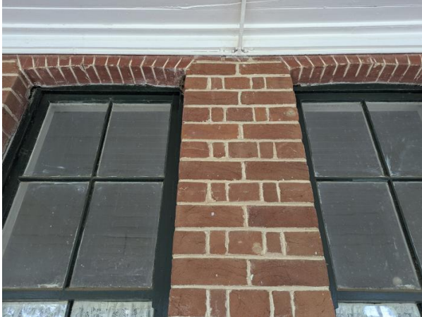
Photo 12 Engineer to advise on remedial work to headers or retain and stabilise
