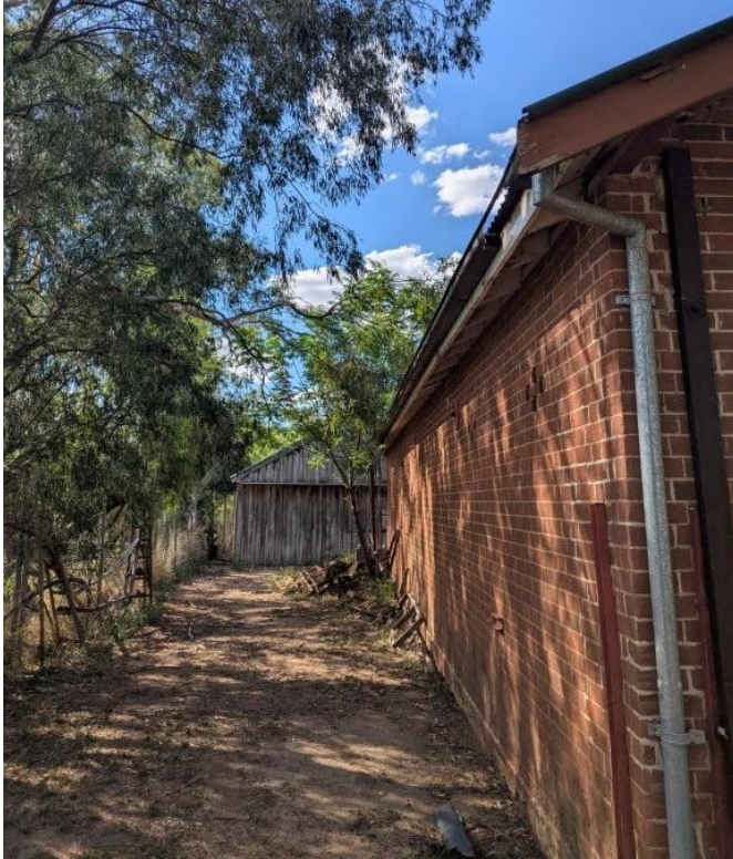
Photo 32 The slope indicates that water ponds against this wall. Note that the gutter is not operable and water drains down the wall from the whole roof.
